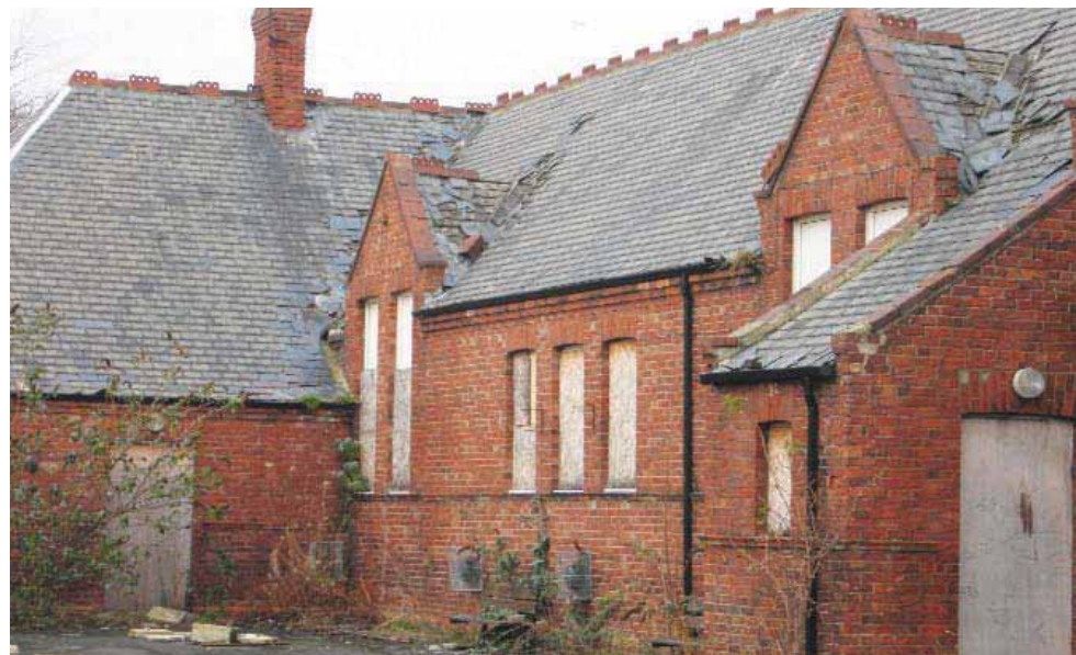
The vacant former village school showing the symptoms of decay and the effects of theft damage, prior to recent repair works being undertaken.
