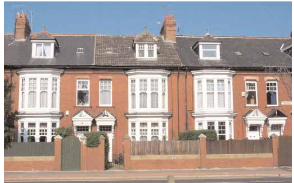
The impact of changing roof materials, (centre), and replacing original timber windows with uPVC (right) or diverting from a colour scheme (porch, far right), on otherwise uniform terraces is detrimental to the special character and appearance of an area.
