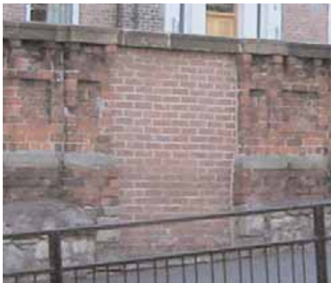
A former opening has been bricked up without regard to the original style, details or materials of the rest of the wall
