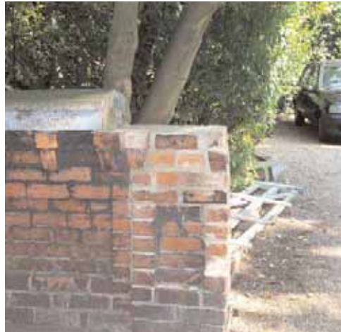
A gate pier missing its decorative capping stone
